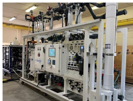
Industrial scale PFAS testing installation at a utility plant. Source: Hazen and Sawyer .
